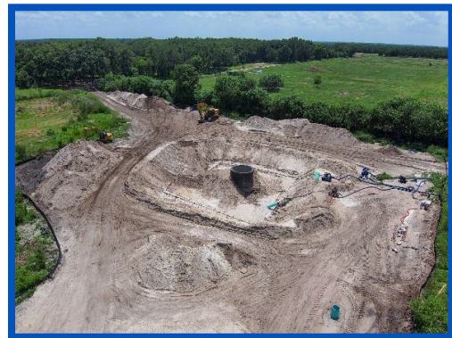
Pace Road Master Lift Station Site.
