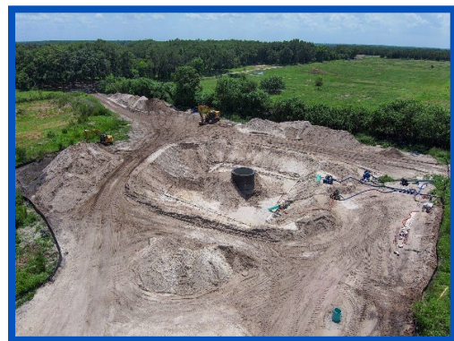
Pace Road Master Lift Station Site.
